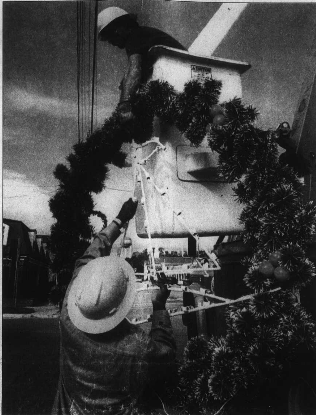
It's beginning to look a lot like Christmas all through the community, with street decorations going up, house lights brightening our evenings and store windows cheering our days. This weekend provides the big kickoff to Christmas-by-the-Sea with the Oak Island holiday parade starting at 3 p.m.
