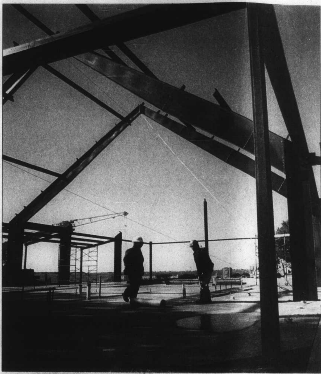
Over the past week steel has virtually leapt out of the ground, and the waterfront skyline has been drastically altered by the Southport community building project. The All-Span Building Systems crew installed the last major roofing support Tuesday.
