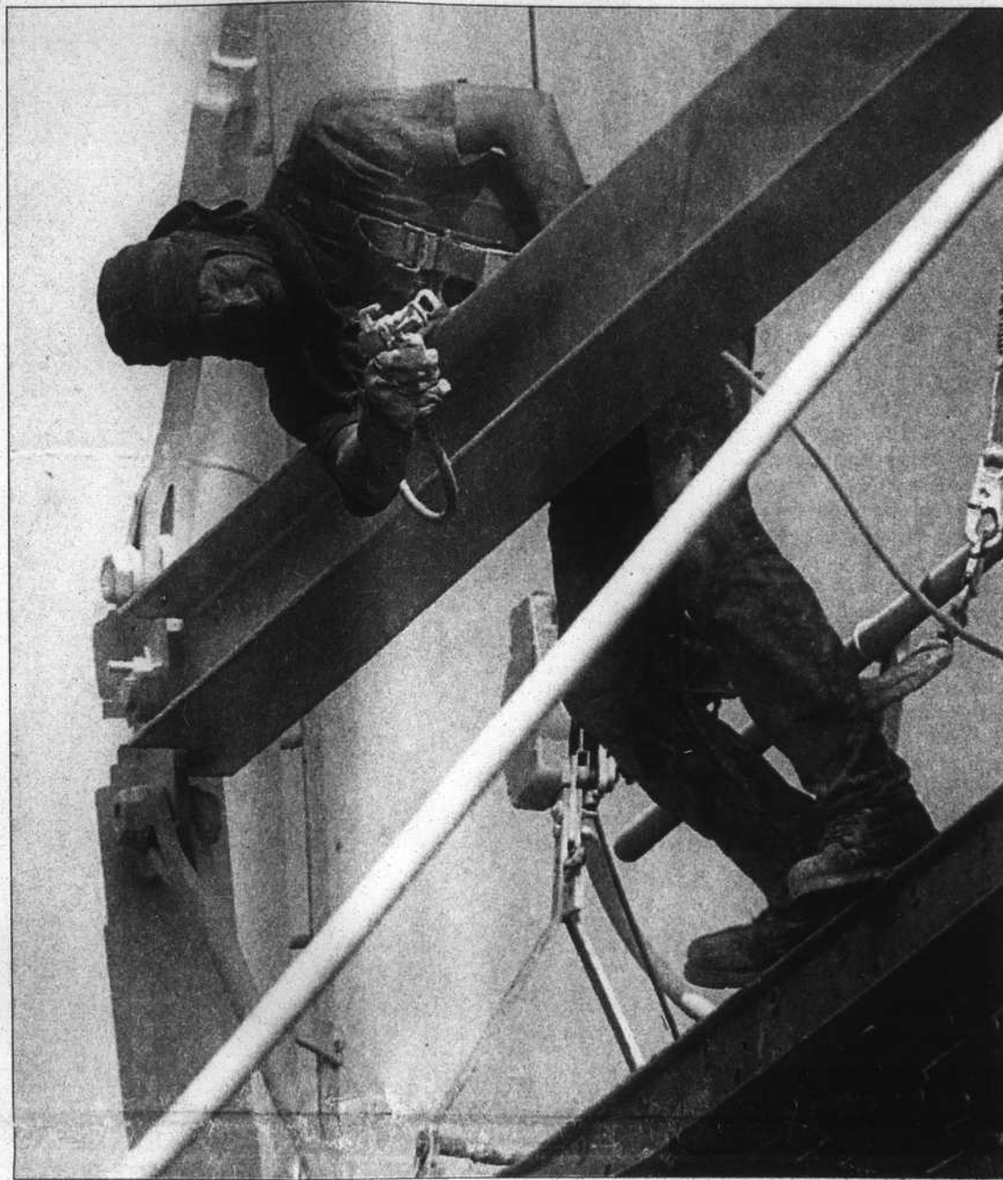
This hooded figure is Shane Kingery, member of a three-man crew from Southern Corrosion finishing up the paint job on the Southport water tower on Sunday. In addition to painting, the workers made some welding repairs to the tank.
