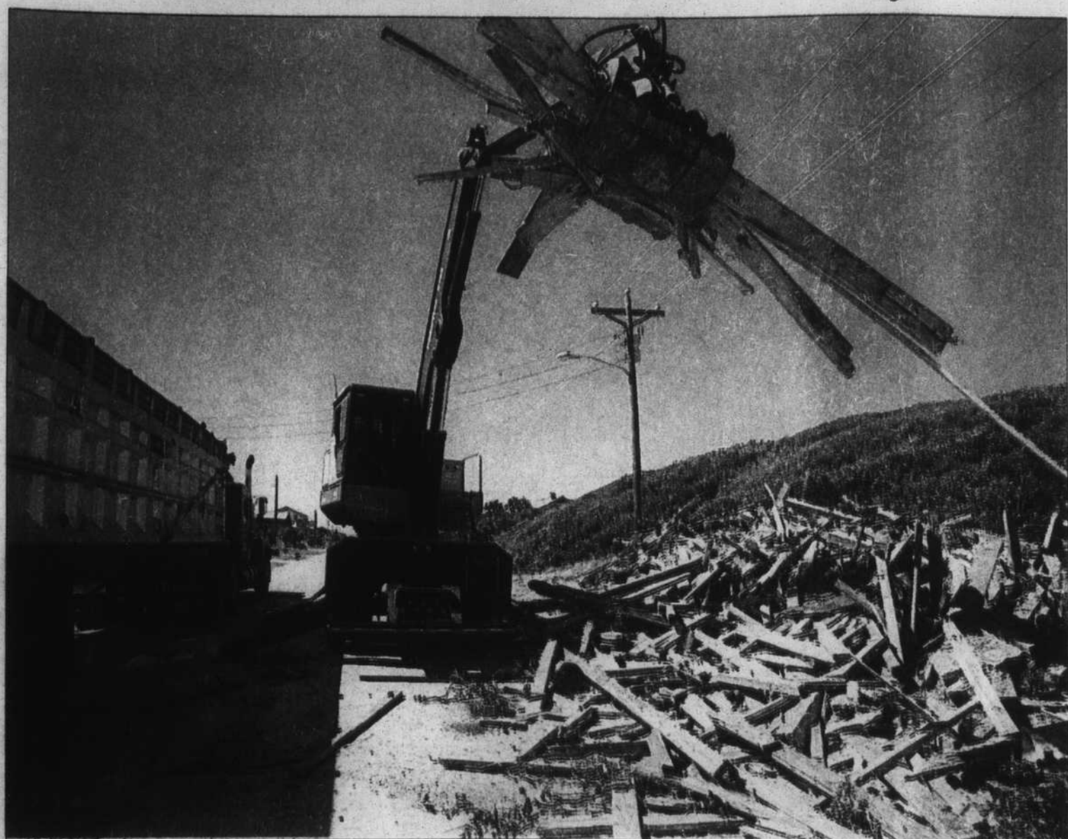
Clean-up of debris from Hurricane Floyd continued along the Oak Island strand this week. Pieces of decks, walkways, porches and cottages were brought to the roadway for loading near 4500 West Beach Drive. The peaked roof in the center background is of one of five Long Beach homes which survived the onslaught of Hurricane Hazel in 1954.
