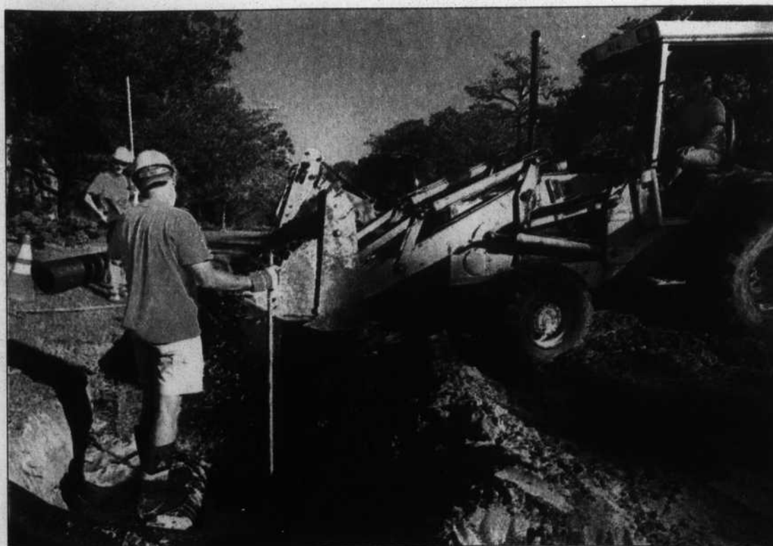
The autumn storms provided challenges in depth for Oak Island's public works department. While cleanup and repair continued last week on the oceanfront, other town workers were installing storm drains where heavy rains had created a flooding problem on 47th Street NE.
