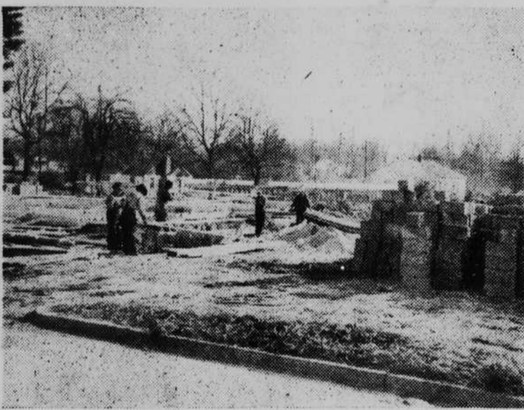
Work is progressing rapidly on the American Legion Memorial building, pictured above, and members of the building committee this week state that a fund raising campaign will be launched in the near future to raise sufficient money to complete the structure. Dedicated to the Transylvania soldiers who lost their lives in World Wars I and II the memorial building is located on East Jordan street on the lot donated by the town. (Staff Photo)
