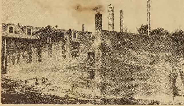
Construction on the new $251,136.00 Harry H. Straus wing to the Transylvania Community hospital is ahead of schedule, and officials of the McMullen Construction company believe the addition will be completed in mid-September. It can be noted in the picture above that construction is nearing the two-story level and the structural steel beams have already been installed. (Times Staff Photo)
