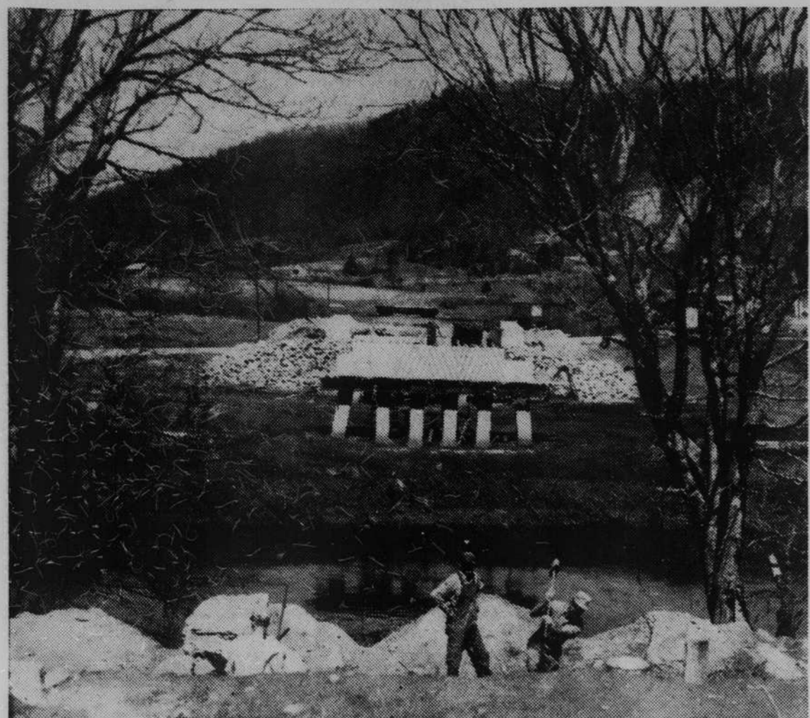
CONSTRUCTION ON THE NEW bridge at Penrose is proceeding on schedule, and when it is completed, the Little River community will be out of the "high water." T. F. Houser company, of Asheville, is the contractor on the project, which calls for the building of five, 57½-foot spans over the French Broad river. Cost of the new bridge is $58,665.10. (Times Staff Photo)
