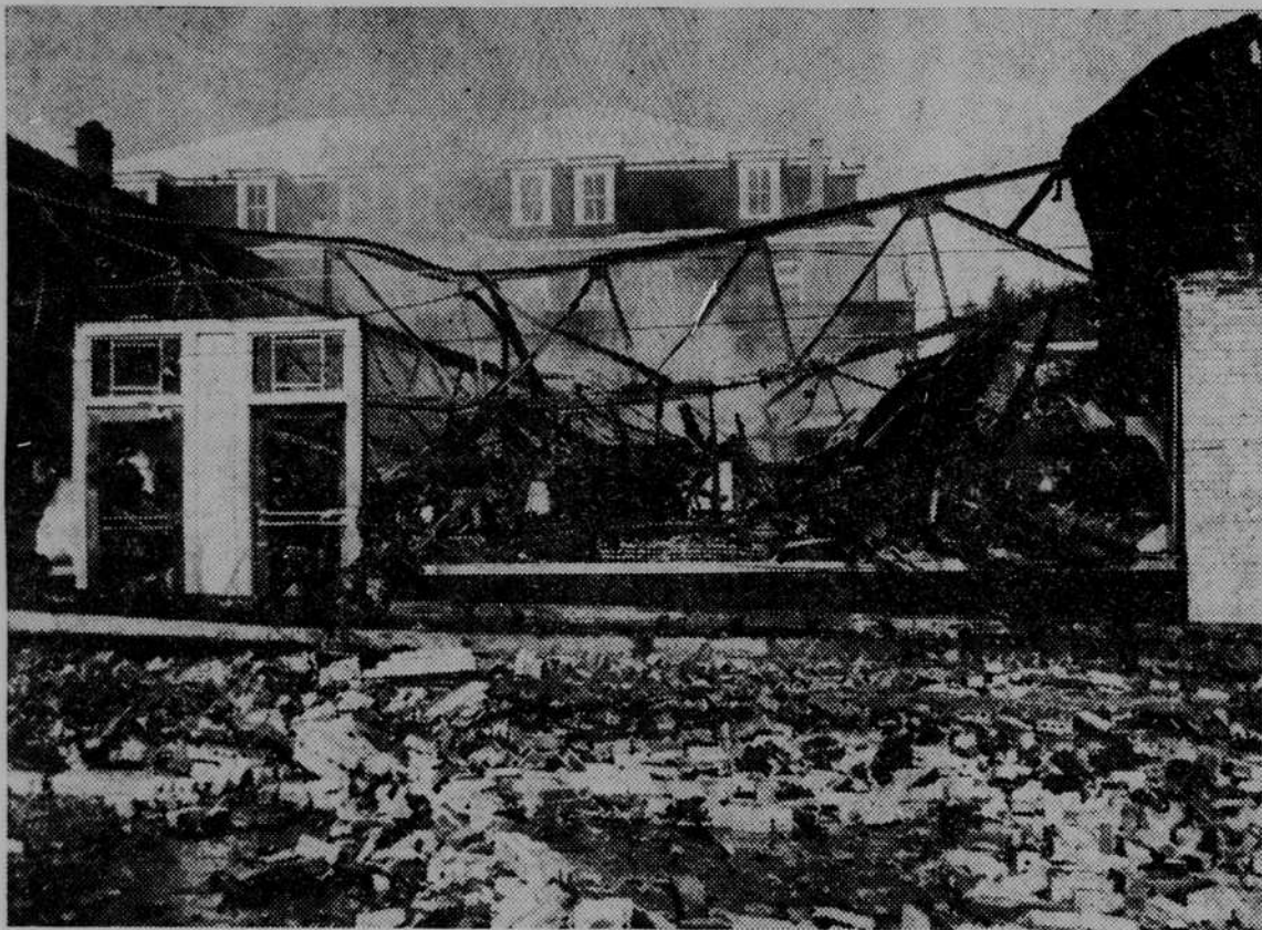
SMOULDERING RUINS, all that remained after the fire at Brevard's A & P Super market last Sunday morning, are pictured above. Broken bricks were scattered all over the street in front of the
