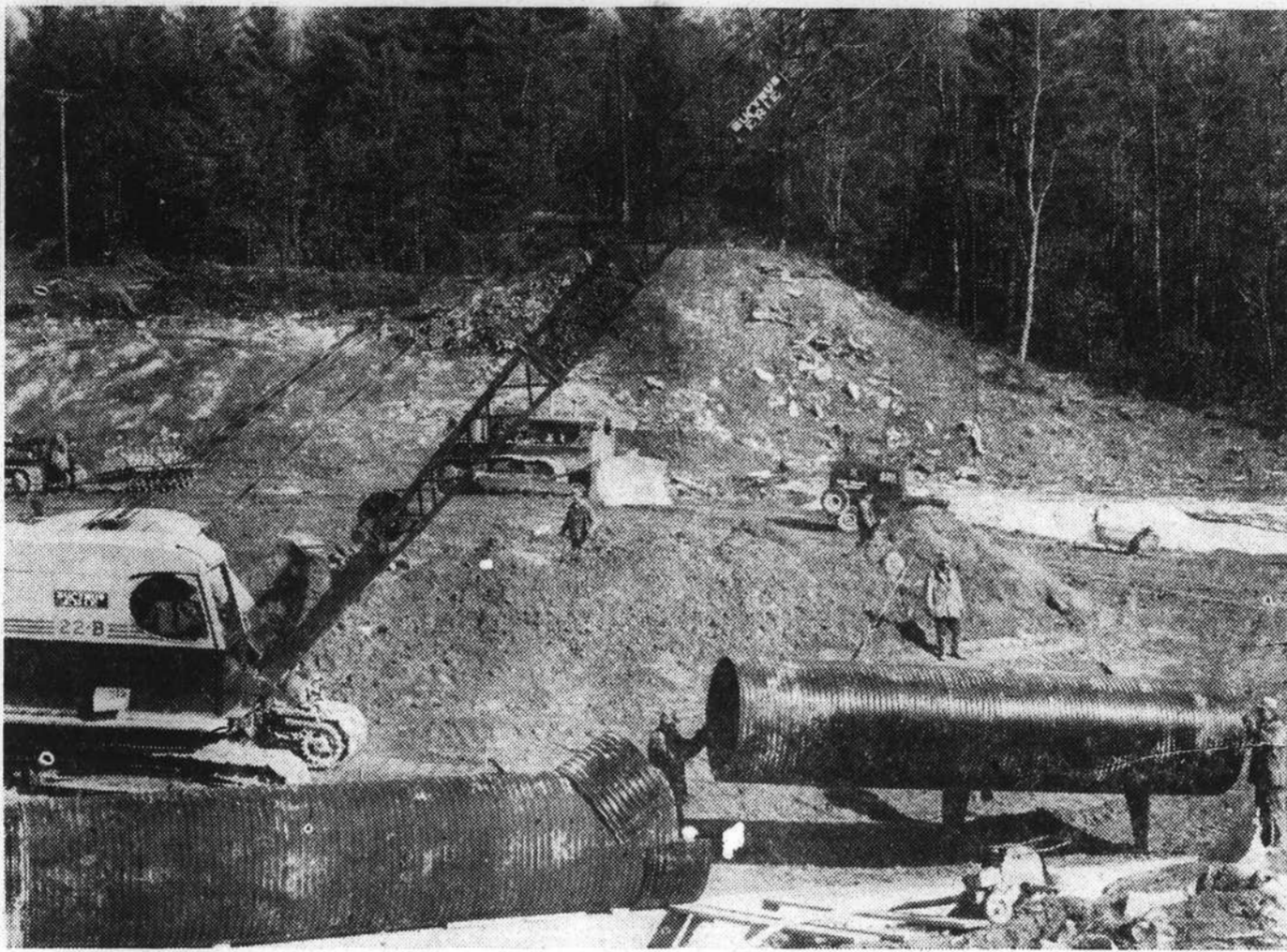
A SECTION of 48-inch corrugated metal pipe is placed in its concrete cradle as construction advances on a dam for new Lake Toxaway in our North Carolina Blue Ridge Mountains. This pipe
