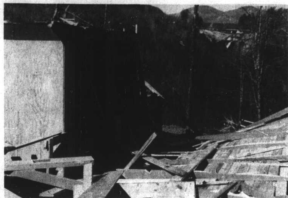
WIND DESTRUCTION — 65 to 100 miles an hour. That's This nearly-completed home at Lake Toxaway was shattered in Thursday's winds estimated from portion of picture. (Times Staff Photo)
