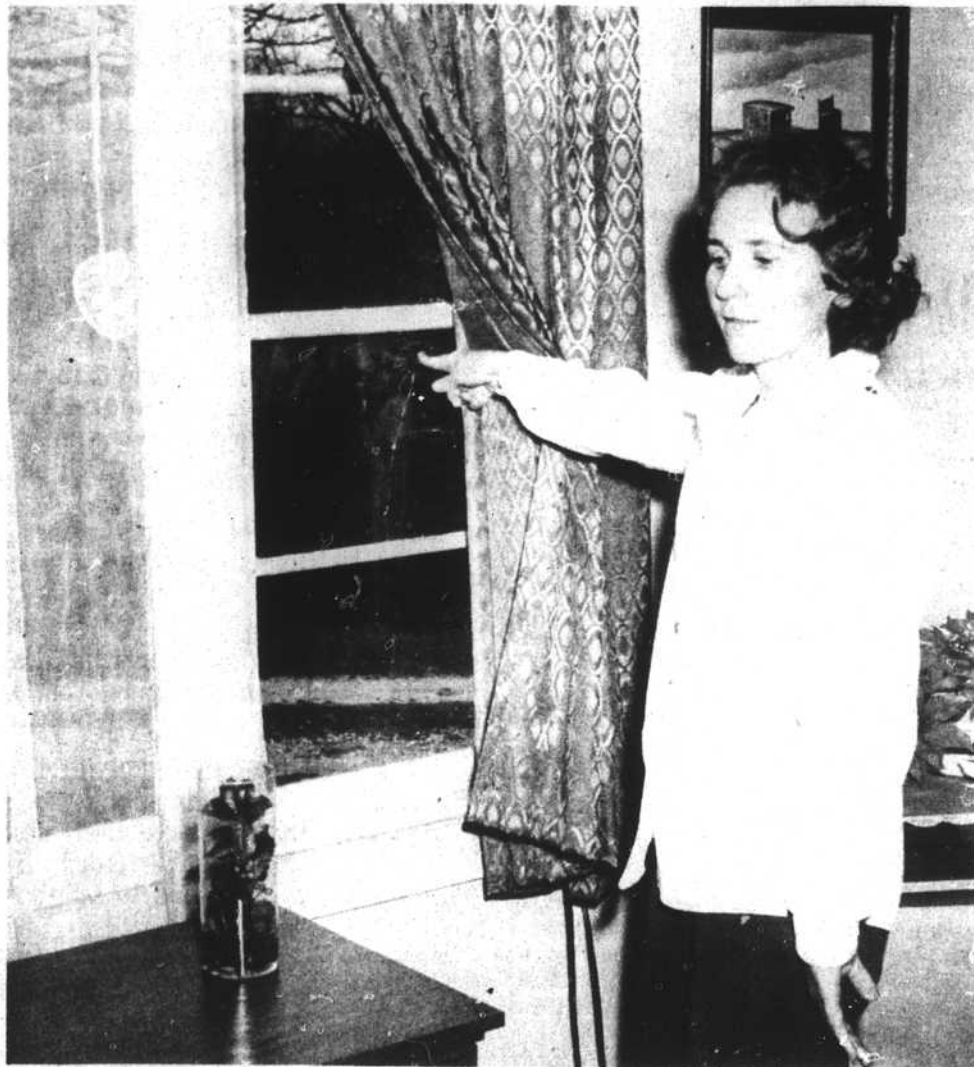
Mrs. Fred Hogsed points out hole where high powered rifle bullet came through the glass of the family living room. (Times Staff Photo)
