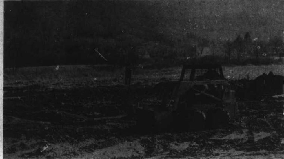
WORK HAS BEGUN on the new Penrose Post Office on Old Highway 64, located about 100 feet behind the present post office. A dirt mover levels site as workman eyes site for foundation of new edifice.
