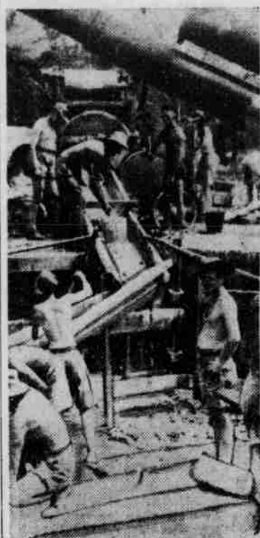
Australian soldiers are pictured concreting a gun emplacement near Darwin, in northern Australia, as they prepare to meet the onslaughts of the invading Japs. This is in the MacArthur theater of operations, where sizeable U. S. fighting forces have joined with their Anzac brothers. Note the colorful campaign hats.
