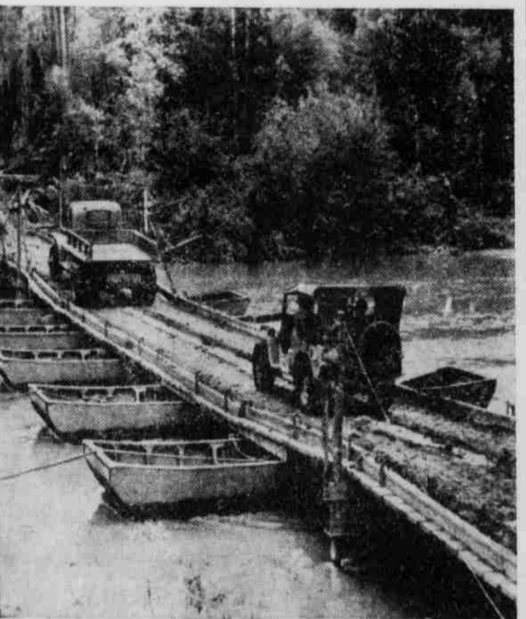
The Alaska highway, which is being rushed to completion through virgin forests on the east side of the Rockies, will make a military road protected by a chain of coastal mountains from the Pacific Northwest to our Alaskan defense area. Photo shows a pontoon bridge over a river. Substantial loads of equipment and supplies may be moved freely over this type of bridge.
