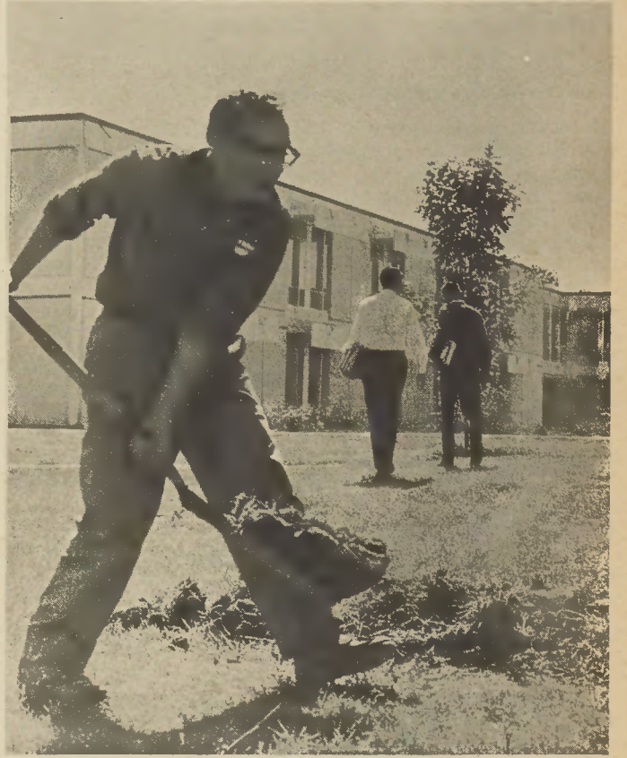
Workman digs in to find leaky pipe.
