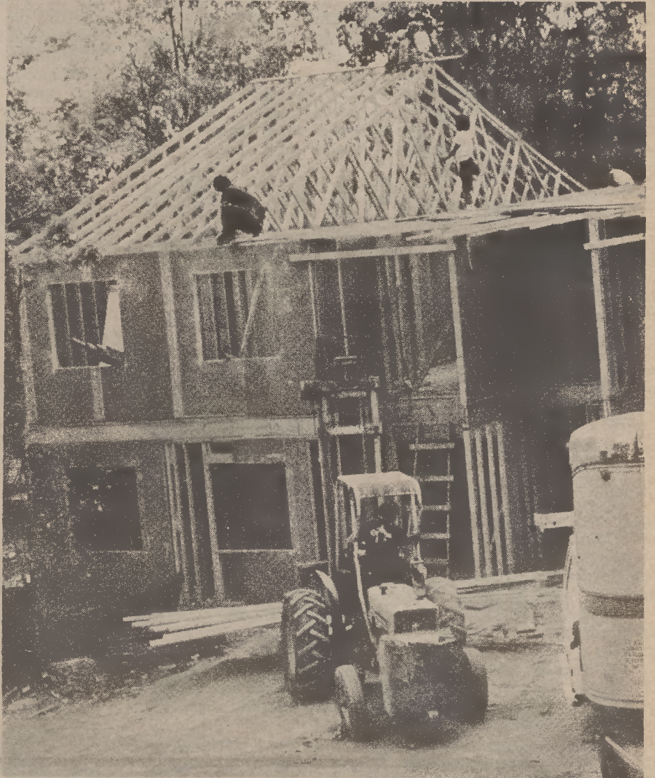
Construction of the new apartment-style dorms behind Holshouser Dorm is right on schedule, according to Residence Life Director Chuck Lynch. photo by Jack Green
