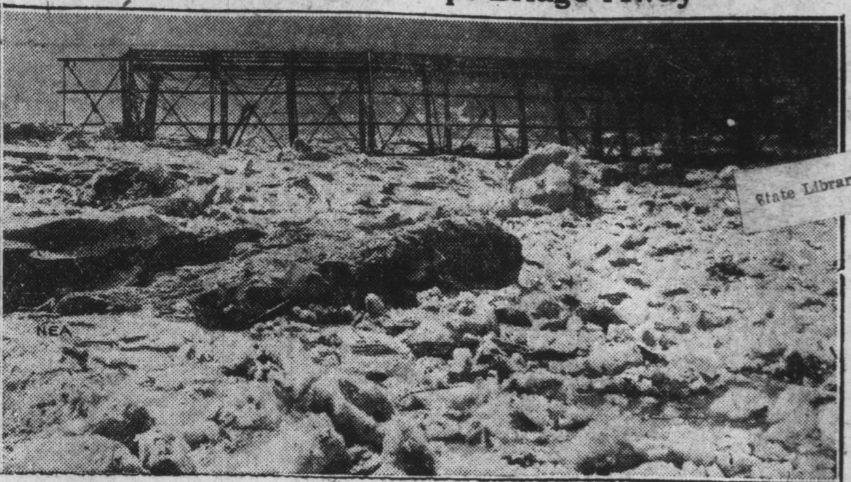
Thousands of tons of ice borne downstream by the flooded Allegheny river at Franklin, Pa., exerted such tremendous pressure that a steel bridge was broken in half and part of it swept away.
