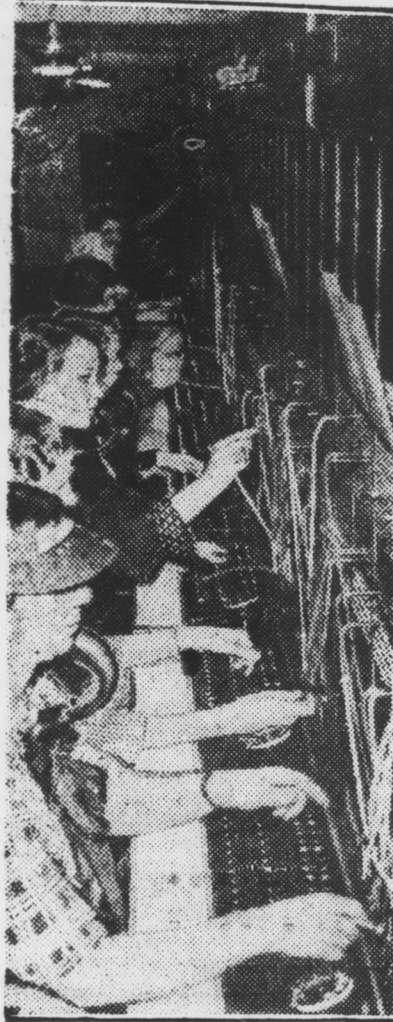
Switchboard at Capitol has been enlarged to take care of expected increase in calls when new Congress convenes, because of larger number of government agencies with which senators and representatives must deal. Congressmen opposed dial system, so this heavy of operators will do the switching. (Central Press.)
