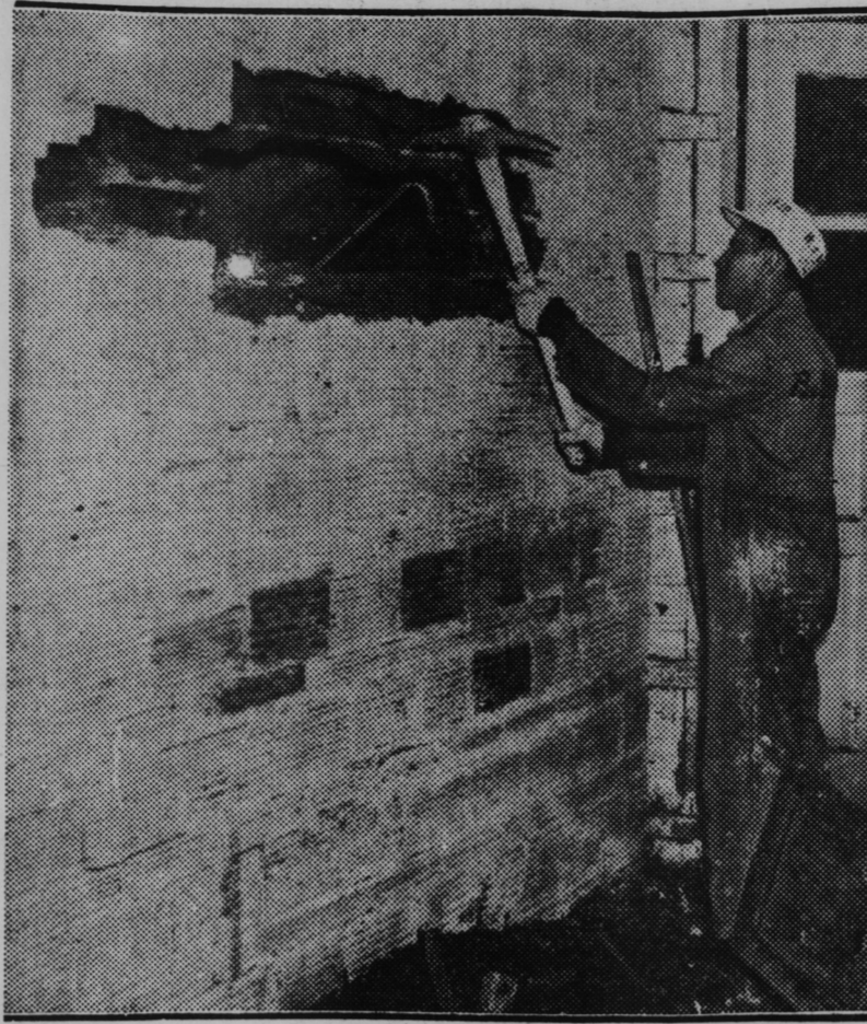
A worker is shown tearing out the wall on the back of the steps of the former home of Gaston B. Means, after a cellmate of the convicted swindler told the police that Means had cached $100,000 in a hollowed-out place under the concrete steps. The money is said to be the sum Means received from Mrs. Evelyn Walsh McLean for the return of the kidnaped Lindbergh baby. The money has not yet been recovered. (Central Press)
