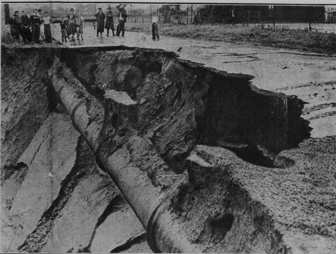
At Wallington, N. J., the steady fall of rain during the last week undermined Maine Avenue, washed away a section of the road and exposed this water main. Many sections of the east, from Maine to Georgia, have suffered from the almost unprecedented rainfall which not only ruined millions of vacations, but caused millions of dollars in damage to property and took several lives. (Central Press)
