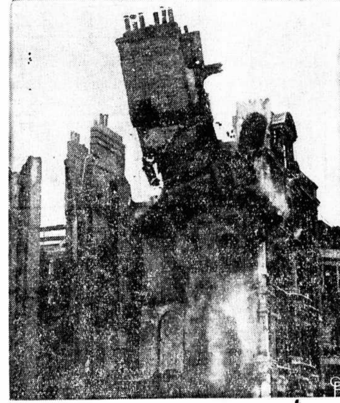
This building was left a mere shattered shell of walls after a raid by Nazi bombing planes. Condemned as unsafe to passers-by, the bomb shattered walls are brought down by a clean-up demolition squad, finishing the work of the aerial invaders.
