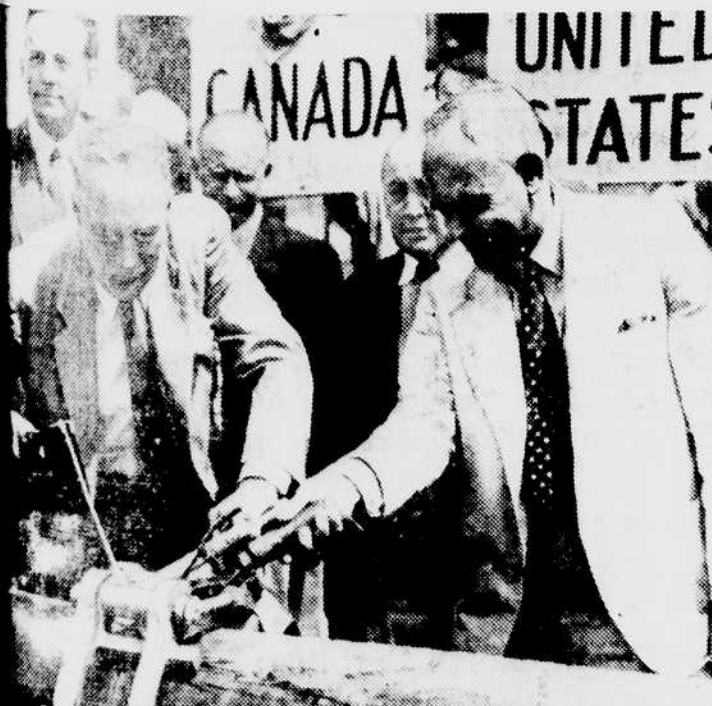
Gov. William H. Willis (left) of Vermont, and Hon. C. D. Howe, Canadian minister of munitions and supply, use teamwork in welding the U. S. and Canadian sections of a 236-mile oil pipeline at the International Border. The pipeline joins a tanker terminal in Portland, Me., with oil refineries in Montreal and will aid in relieving the gasoline shortage on the East Coast. (Central Press)
