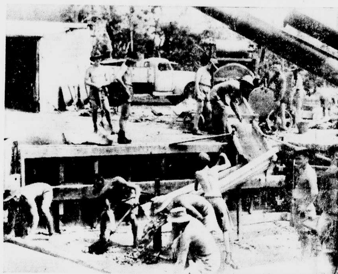
Australian soldiers are shown building a gun emplacement near Darwin, in northern Australia, prepared to meet the expected onslaught of the Japs. This is the MacArthur theatre of operations and already large U. S. fighting forces have joined the United Nations' war effort to prepare the Japs a warm welcome. (Central Press)
