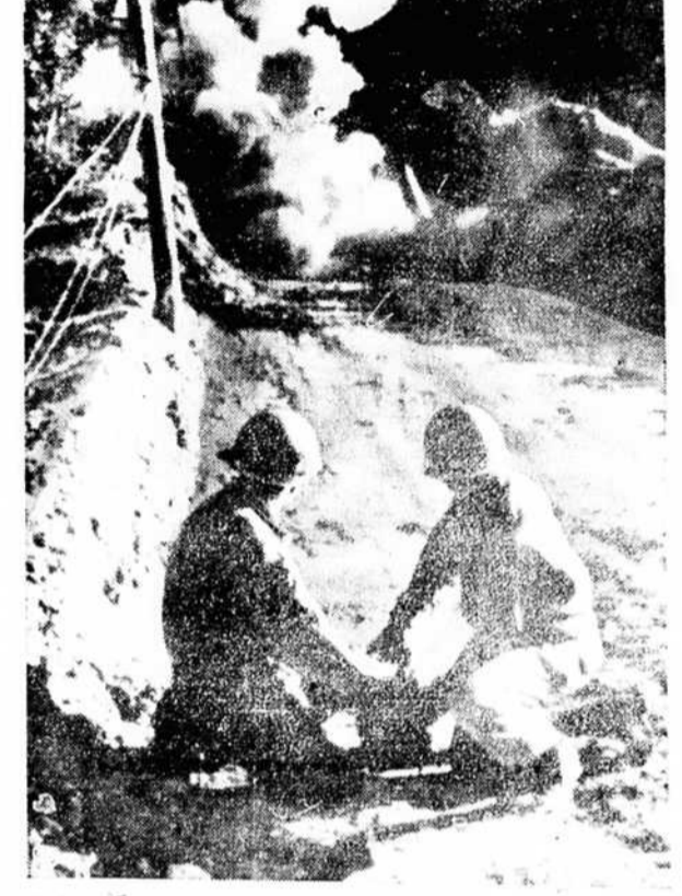
U. S. ENGINEERS blast a highway obstruction in Italy as they prepare to rebuild a culvert that the retreating Nazis destroyed. Much Allied energy has to be spent in this way, merely in order to get through and hit the enemy again. OWI radiophoto. (International)
