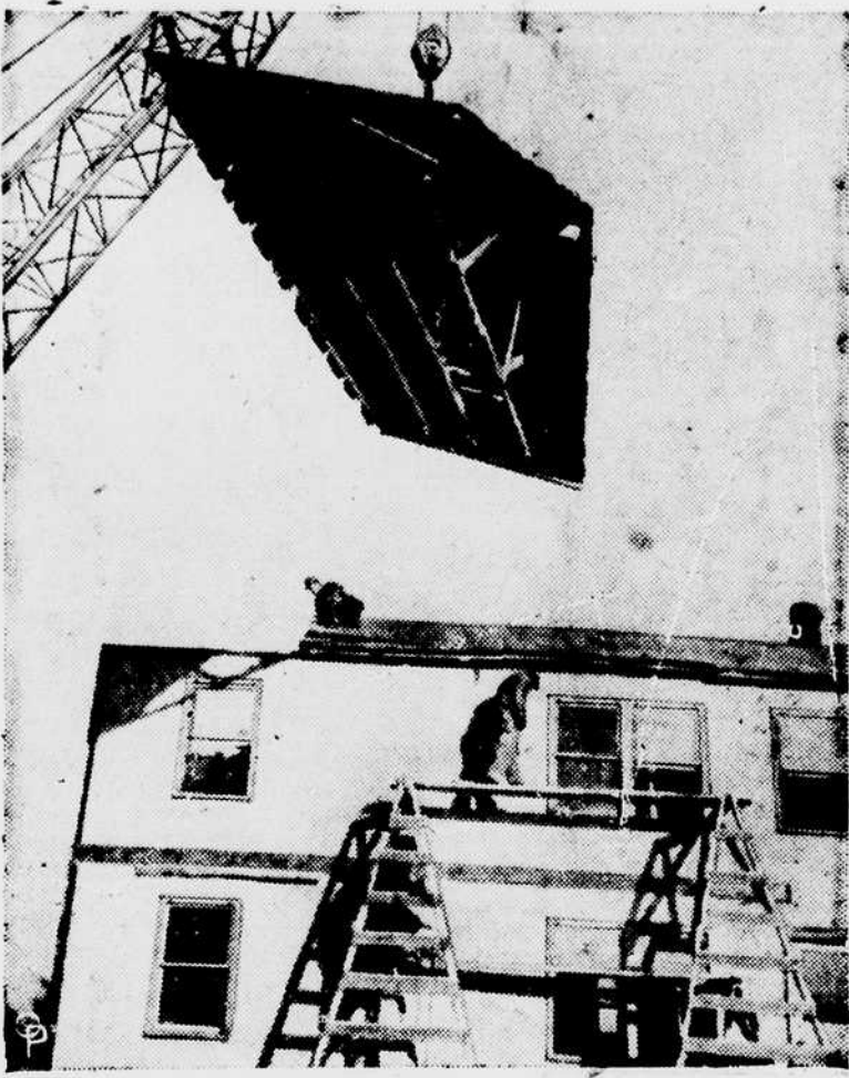
THEY'RE LITERALLY RAISING THE ROOF in East Hartford, Conn., where temporary dwellings, built to accommodate millions of workers in wartime production centers, are being taken apart and shipped to areas where the housing shortage is most acute. A huge crane is shown lifting a section of a two-story house, which will be one of 2,000 to be put together again for returned vets in the New York area. (International)
