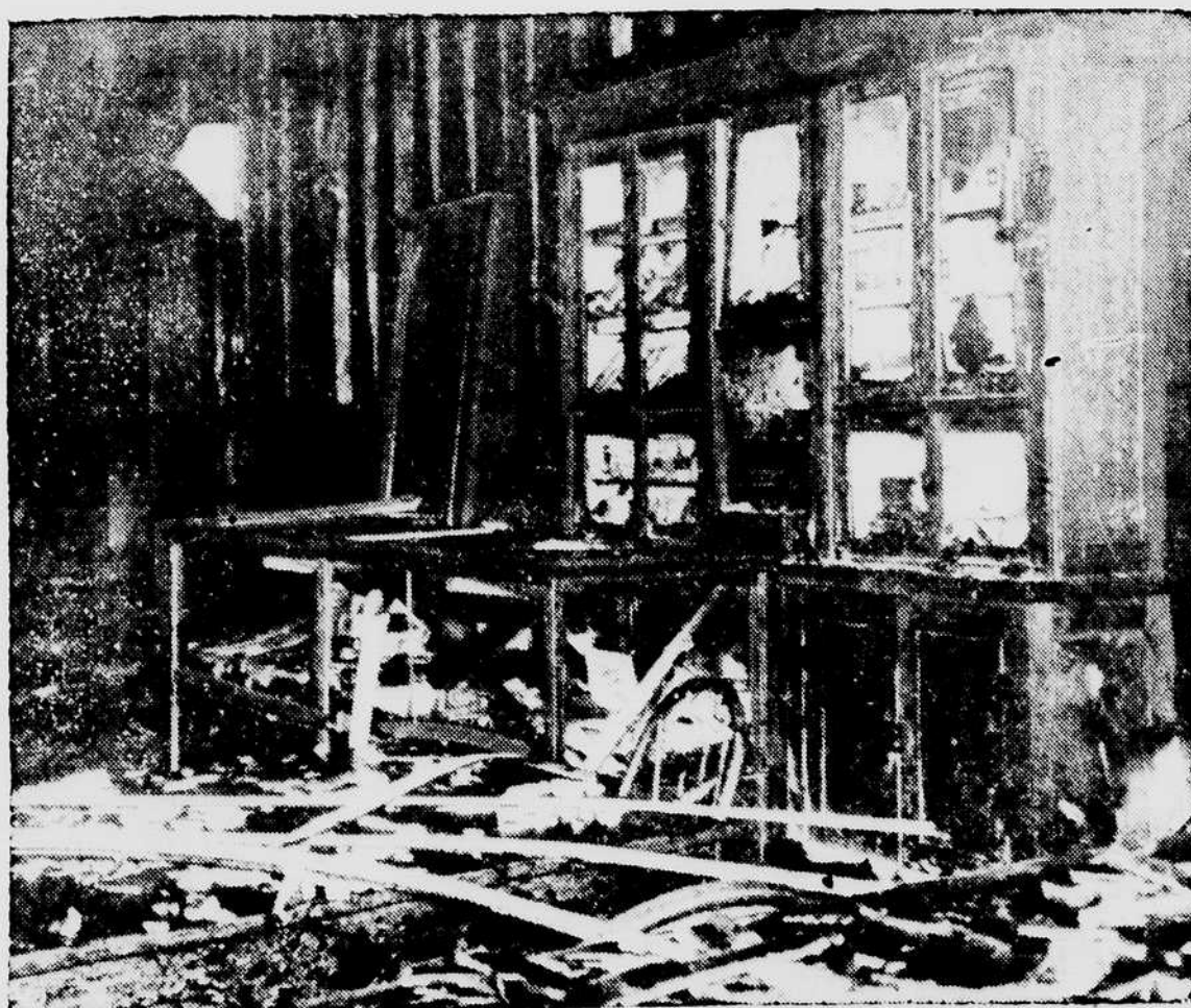
CHARRED debris is scattered through the burned-out lobby of the 50-year-old Canfield Hotel in Dubuque, Iowa, where 16 persons lost their lives in a fire which destroyed the inside of the hotel. More than a score were injured. The fire started in the older 4-story section of the hotel and spread rapidly through the building and its six-story annex. (International Soundphoto)
