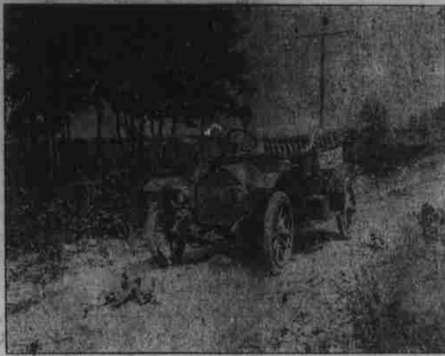
Fig. 5. A road where surface contains a great many stumps. Such a road cannot be maintained properly.
