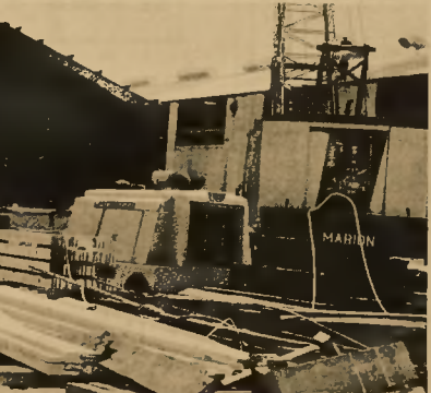
Company in Murfreesboro, who recently merged with Georgia-Pacific Corporation, is completed. Work is well underway with the cost of the expansion to be in the neighborhood of $1.5 million.
