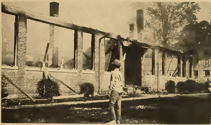
NOT MUCH LEFT — The charred skeleton was about all left standing as firemen continued to fight the blaze of unknown origin which broke out early Saturday in the abandoned Mars Hill School at Trap, described as "one of the better buildings in
