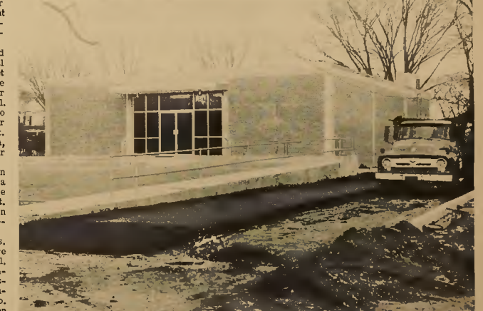
WORKERS BEGAN PAVING the drive at the new Rich Square Post Office Wednesday. Scheduled to begin earlier this week, the work was hampered by rains. Postal officials hope the paving will be completed by the end of this week.
