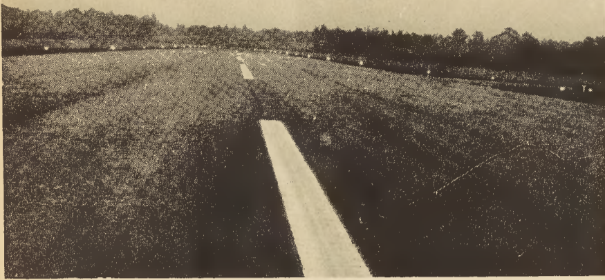
ON AGAIN, OFF AGAIN is the situation regarding the runway lights at Tri-County Airport where lights have been turned on at night by an electronic device despite the lack of obstruction lights which have been held up due to the heavy rains making it impossible to get into area with
