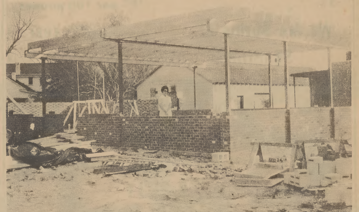
NEW RICH SQUARE EATING PLACE — Mrs. H. C. Simmons Jr. of Woodland looks over the construction of a new drive-in restaurant she and her husband are building. It will be designed along similar lines of their other Northampton
