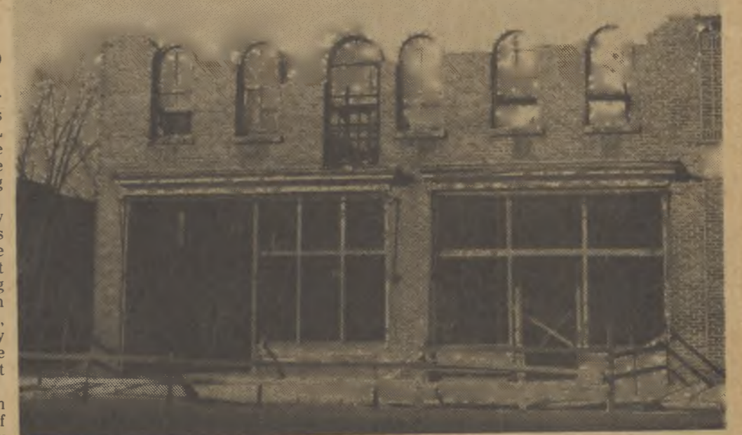
DOWNTOWN JACKSON IS taking on a new look as an old derelict is taken down to make way for a new building for the Northampton County Farm Bureau. The new structure will be of Colonial design and plans call for completion by the fall.
