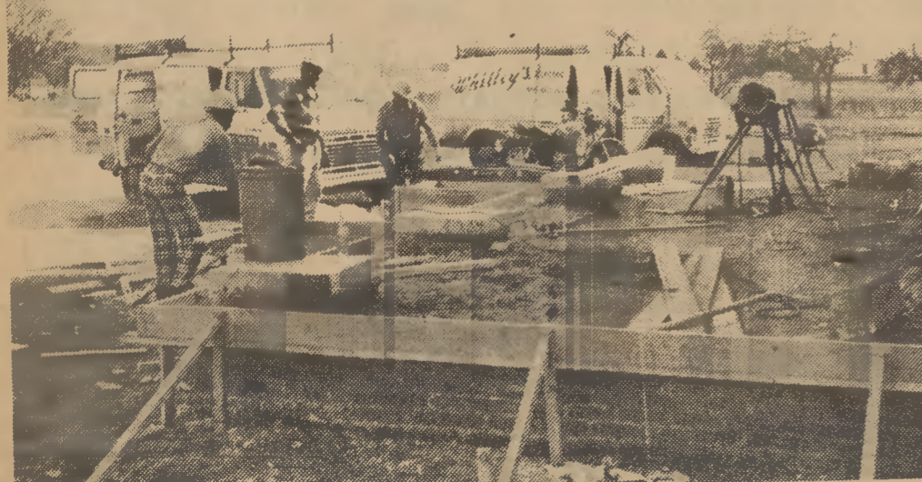
A NEW FRONT PORCH ON THE Old County Home is attended to by Roscoe Howel, John Sledge and A. G. Berguson. Progress on the renovation of the home is going along on schedule and plans call for completion in the summer.
