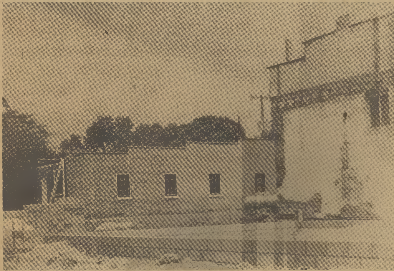
THE FOUNDATION IS NOW BEING LAID for the new Farm Bureau office. Rainy weather and muddy ground have slowed the building process but now that the sun is out more often, progress
