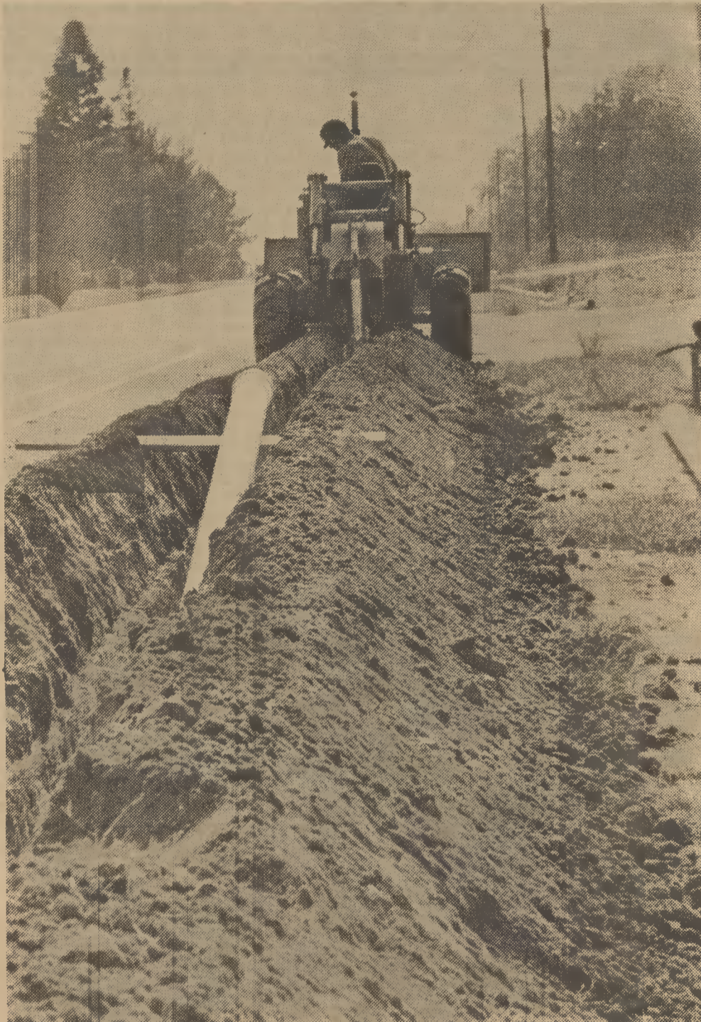
WORKMEN FROM Connell Construction Co. in Warrenton are busy planting water mains along U. S. 301 in Garysburg. The project is being undertaken by the Progressive Garysburg Water Association at a cost of $129,000.
