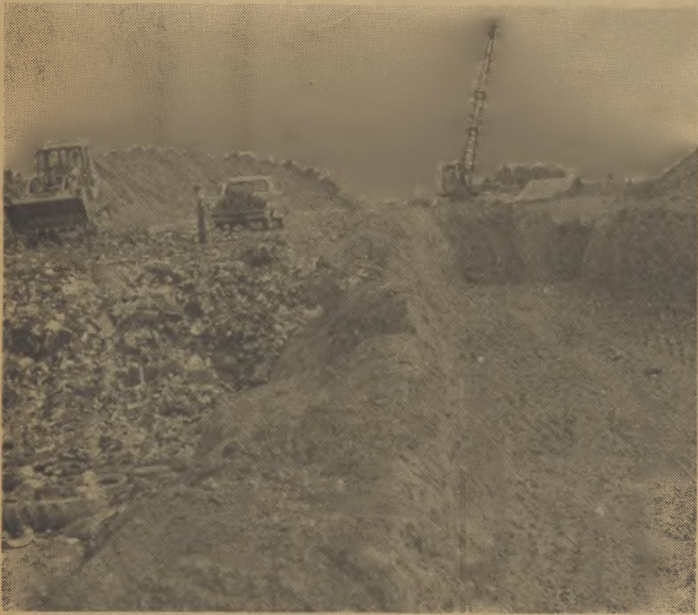
THIRD TRENCH — A drag line trenches another ditch at the county landfill north of Jackson. The 15,000 cubic yard ditch is the largest of the three trenches dug to date. Landfill employees cover daily refuse deposits at left.
