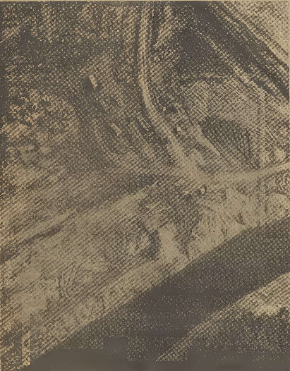
ALBEMARLE PROJECT — Work is continuing on the Northampton side of Roanoke River on the Albemarle Paper Co. water pollution abatement project. The $2.5 million project, which is in Gaston, represents only a portion of the pollution control program underway at the Roanoke Rapids paper mill. The body of water at the bottom of the aerial photo is a tributary of the Roanoke known as Little River.
