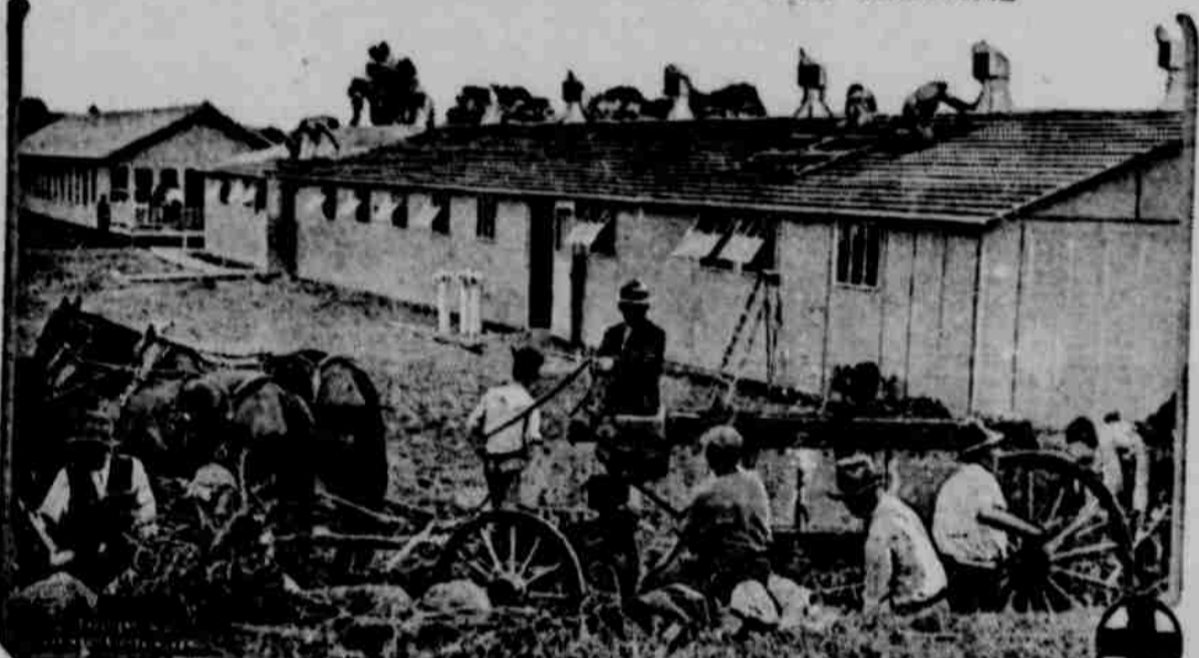
Rushing the work on the Columbia University War hospital in New York city, the first to be built in this country. The hospital will contain 500 beds and will cost approximately $250,000. It is being built on plans which are based on those drawn by physicians and other experts who have had experience in hospital planning with the English and French abroad, and provides for an entirely portable building which in case of emergency can be sent overseas or to any part of the United States.
