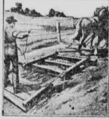
The Spiked Forward Part of the Drag Loosens the Road Soil, and the Following Rear Portion Packs it to a Smooth Surface, Thus Finishing the Surface in One Operation.
