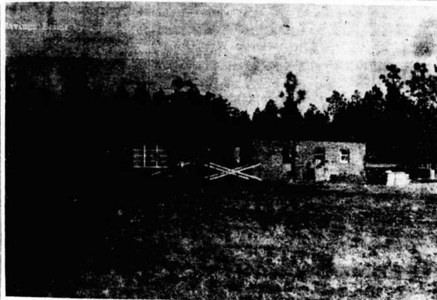
CLUBHOUSE NEAR COMPLETION—Construction of the new clubhouse for the Carolinas Country Club is nearing completion. Preston Hennies, golf pro, estimated that 10 more working days would be required to complete outside construction. The golf course is expected to be opened in early Spring.
