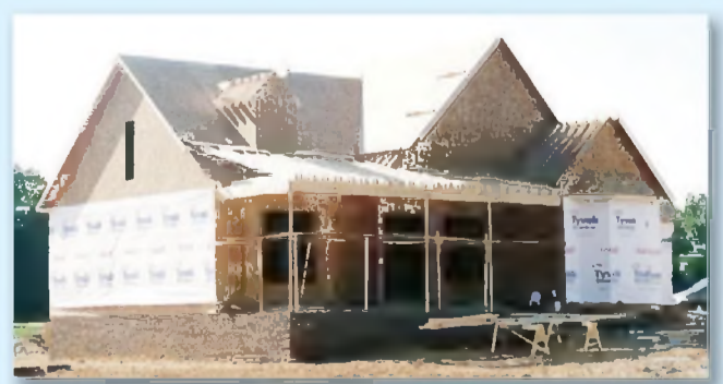
Under Construction - Custom Built Energy Star Home with Sealed and Conditioned Crawl Space
