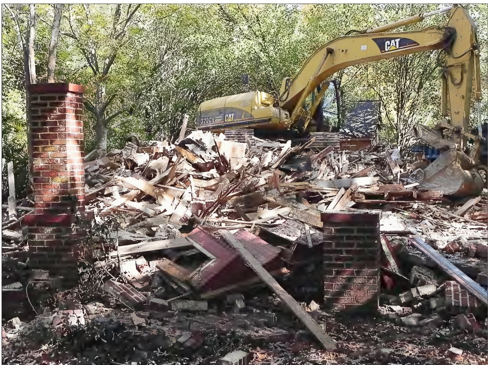
Crews demolished the former Kirby house at the intersection of Ridge Road and Chub Lake Street this week in preparation for a turning lane and traffic light at the intersection.
