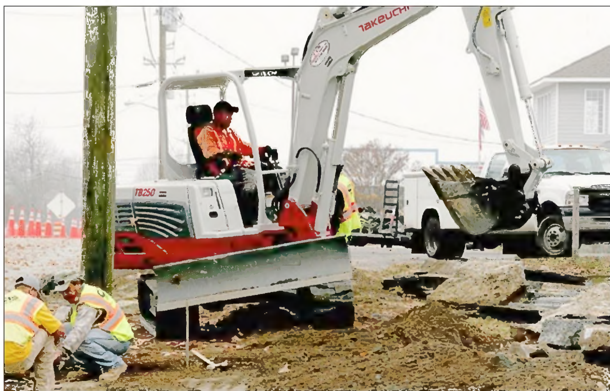
Work on the North Main Street sidewalk construction project continued this week. McQueen Construction, which was contracted to perform the work, estimates the work will be completed by January.
