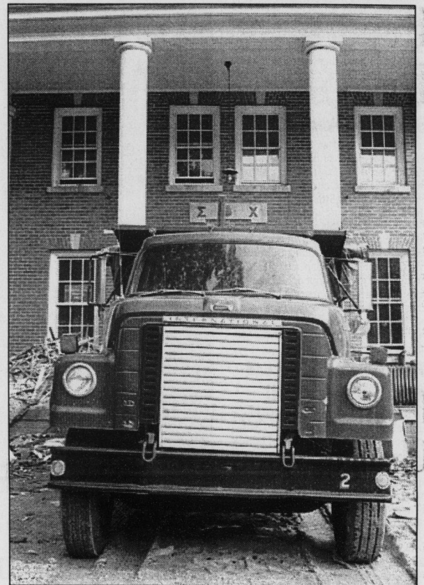
The Sigma Chi house in Fraternity Court is undergoing renovations and expansion this summer. The construction should be finished in the fall.
