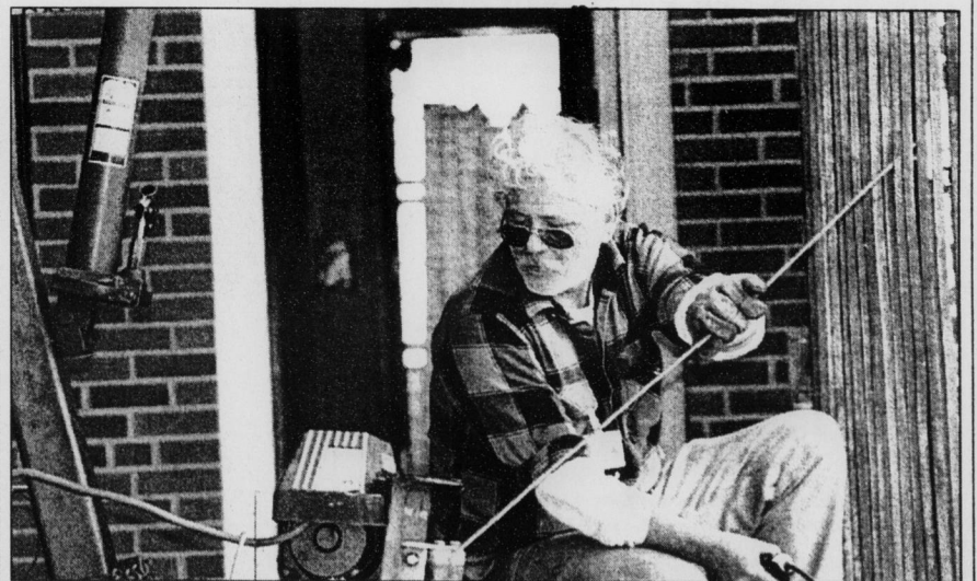
Construction worker John Hundley helps with cable installation on the 10th floor of Hinton James on Wednesday afternoon. Residents should expect to see John and his co-workers for the rest of the semester.
