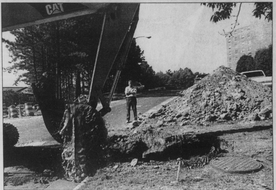
Orange Water and Sewer Authority workers clean up water that burst from the main water pipe Monday beside Hinton James Residence Hall.
