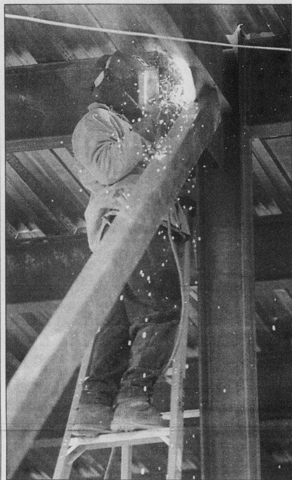
Roger Smithfield welds steel girders at a construction site on Rosemary Street on Thursday afternoon. Units in the building will be rented out as apartments.
