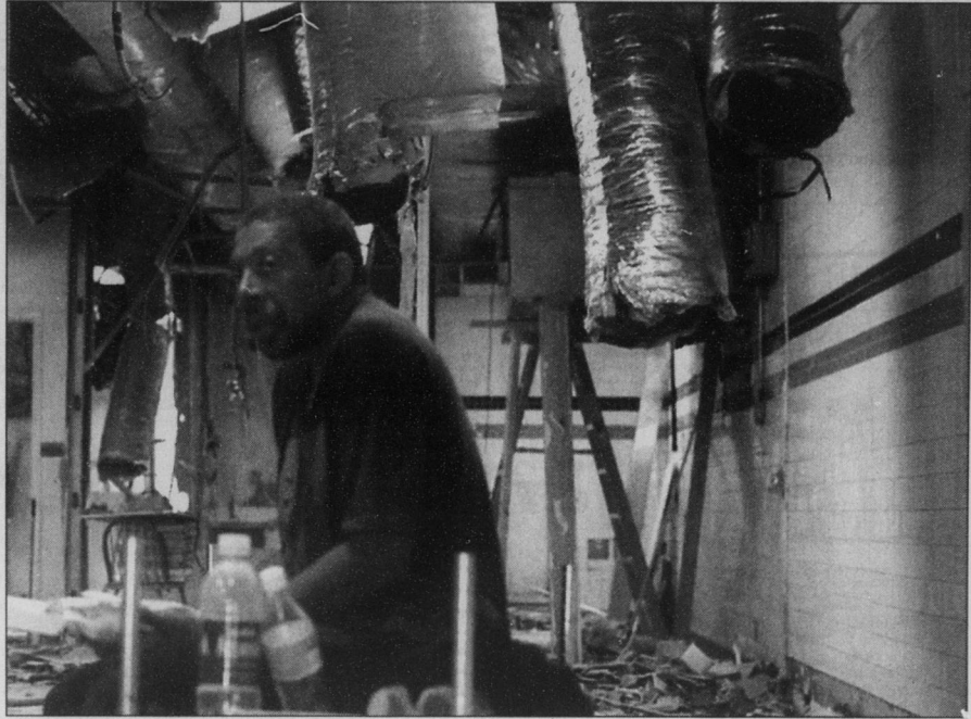
Kenneth Smith of Chapel Hill takes a break to eat lunch while working on the renovation of what used to be Taco Bell on Franklin Street. The building soon will house a women's clothing store.
